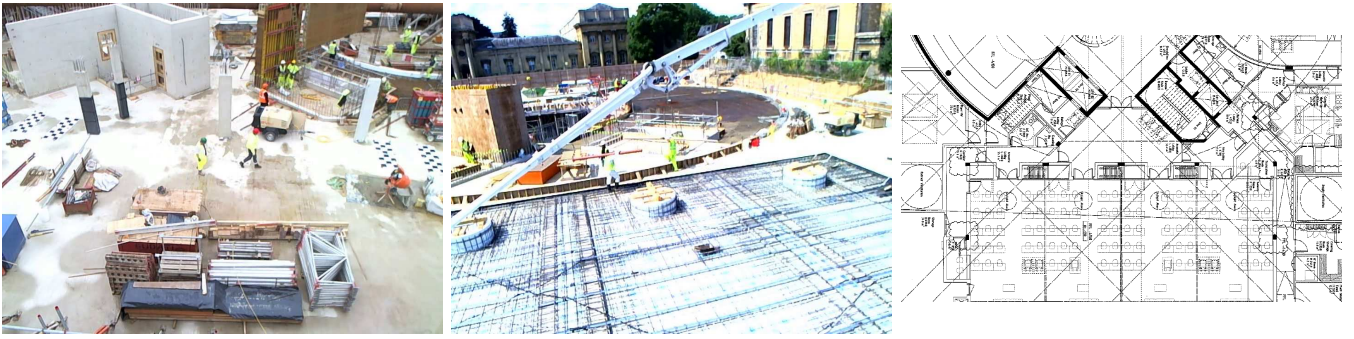
Figure 2: We have conducted tracking experiments in a construction site setting: (a) the construction site on day 1, (b) the construction site on day 36, (c) floor plan of the site. The site changes rapidly from day to day, precluding the use of positioning systems which rely on stable, long-term maps.
